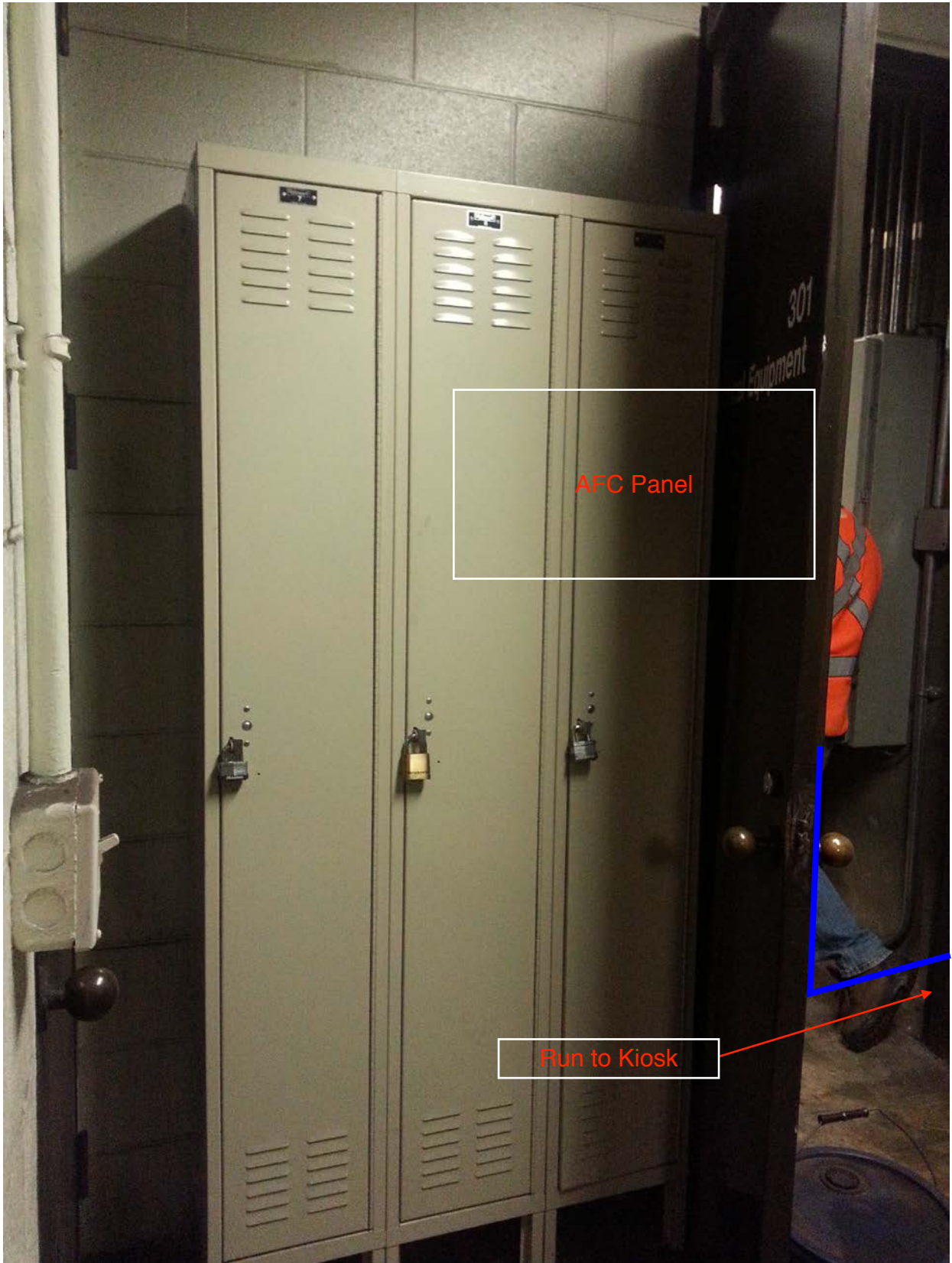
Photo #2 – F06 Anacostia North: Room 301 with AFC Panel NSF
